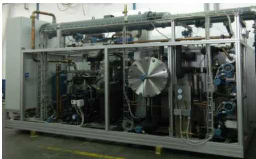
Fig 3: A photo of the whole Cold Energy test bench
